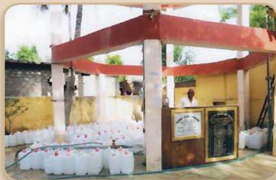
Overhead water tank & treated drinking water supply system managed by the Water Committee in Gangadevapalli
