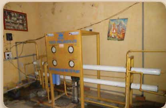
Water Purification Plant funded by Tata Projects from which all households get drinking water in Gangadevapalli
