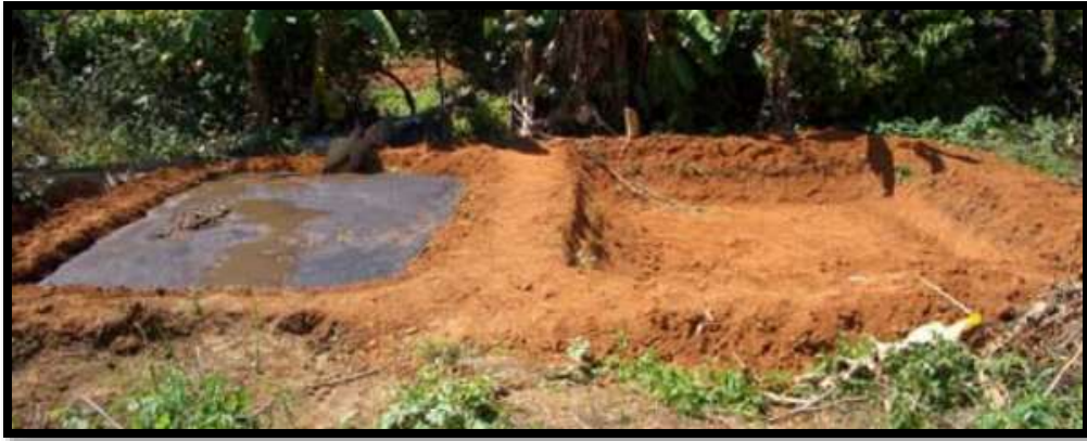
Fig. 7.3 View of simple sludge drying beds
