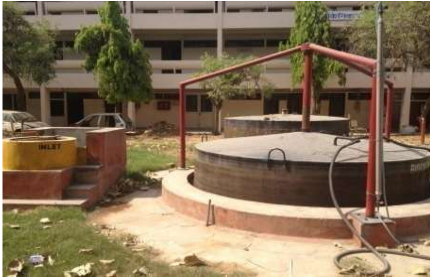
Fig. 2.1 Floating Dome type biogas Plant at IIT Delhi
