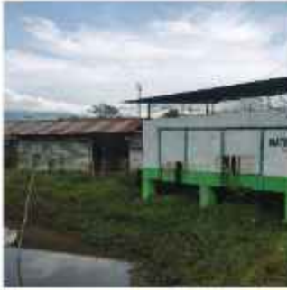
1000 L WATER TREATMENT PLANT BASED ON ROUGHING AND BIOSAND FILTERS
