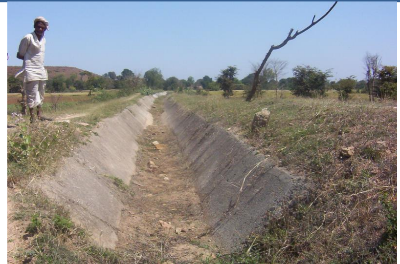
Lined Minor Canal with Silt and Damage
