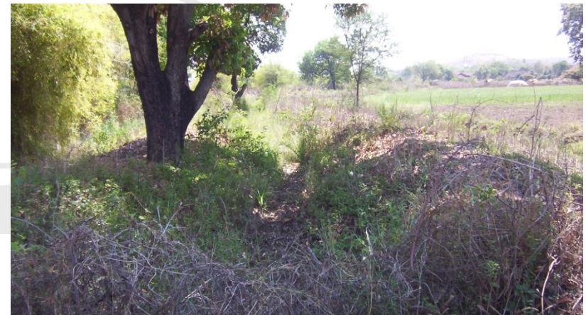
Heavy Weed Growth in Canal Bed
