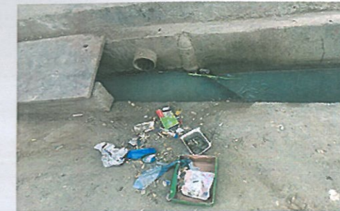
THE BIGGEST PROBLEM OF THE VILLAGE IS SANITATION . ALL THE DRAINS ARE OVERFLOWING AND NO HELP FROM GOVERNMENT IS THERE FOR THE PEOPLE.
