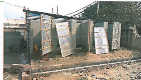
TOILETS FOR THE TEMPORARY STEEL HOUSES.
