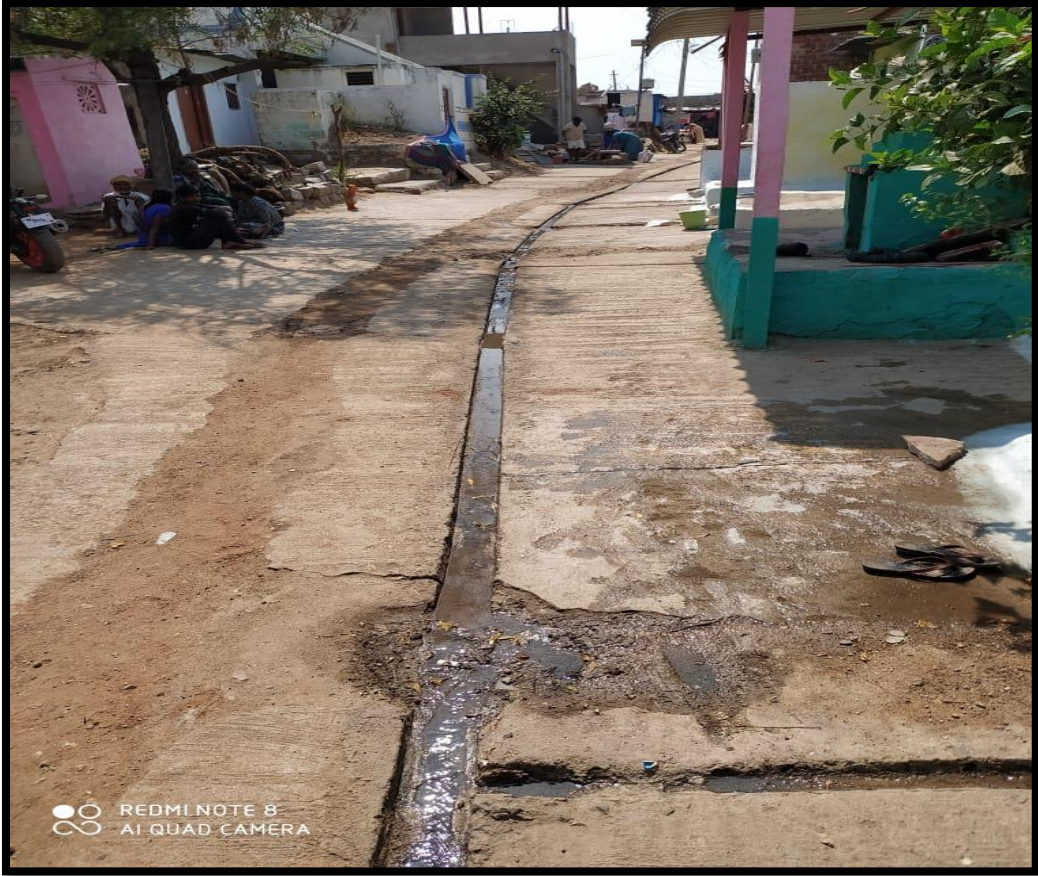
Open Drainages causing lots of Health Issues
