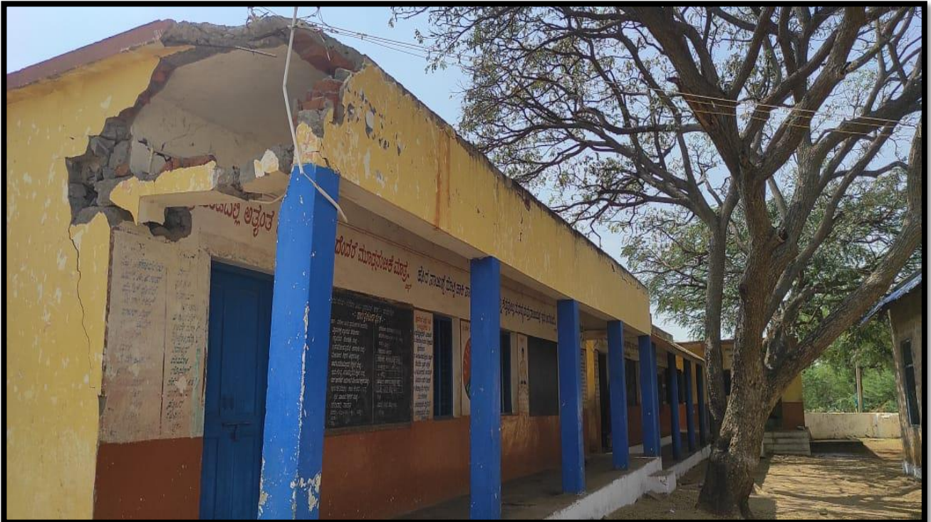
Primary School Building has to be repaired
