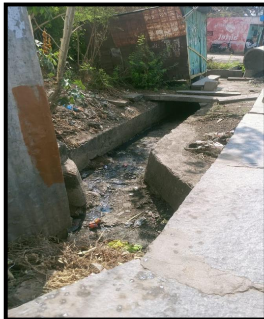
Open drainage system found as LPG
