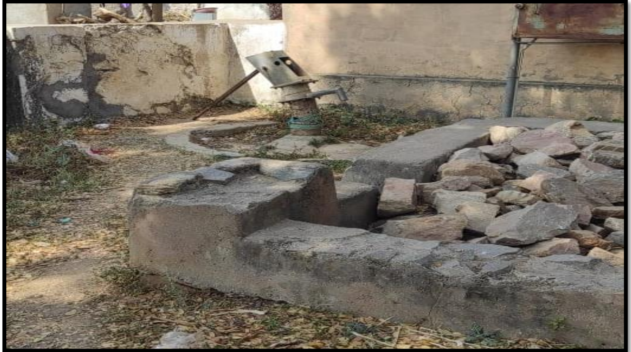
Many hand pumps are not working properly
