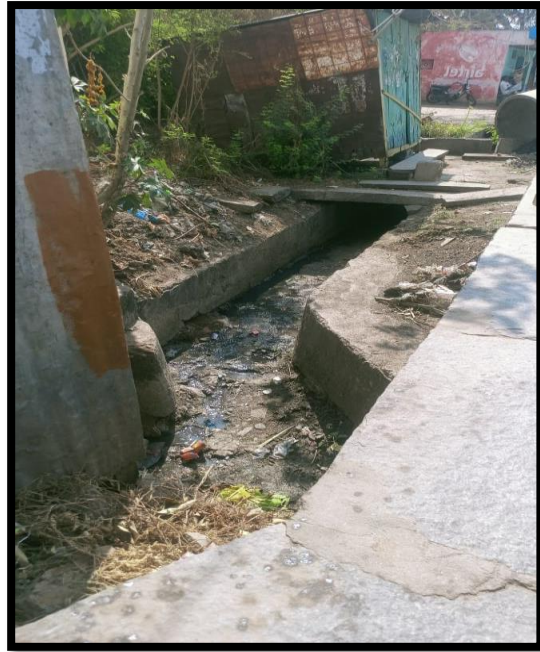
Open drainage system found
