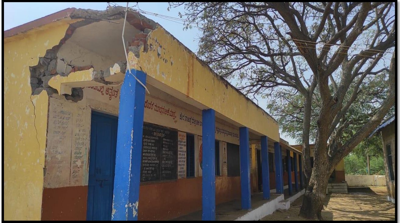
Primary School Building has to be repaired
