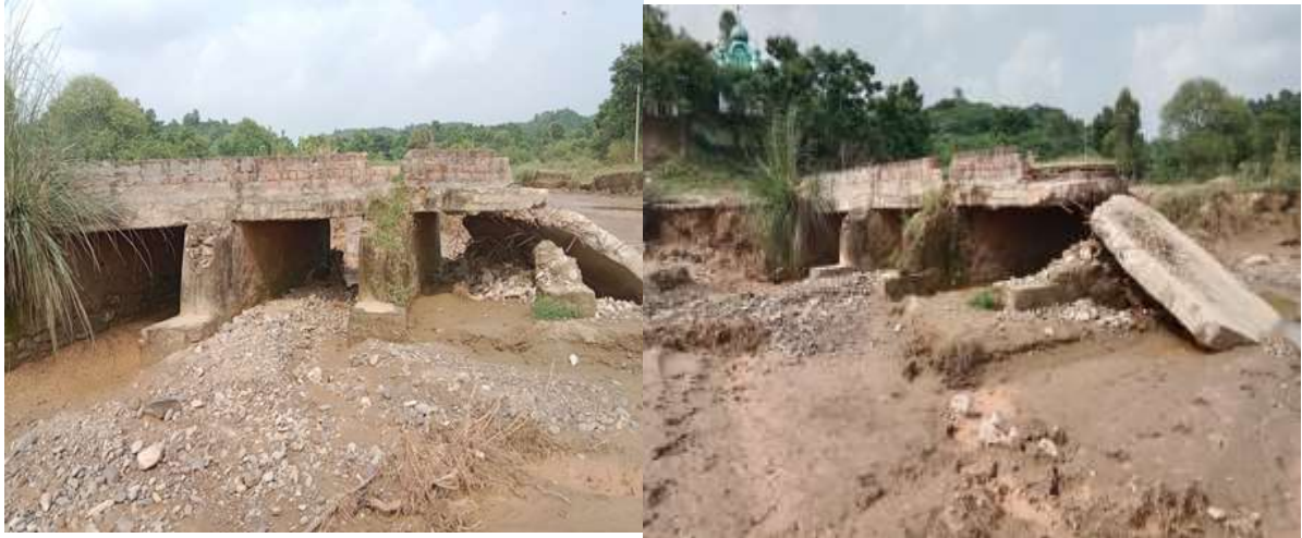
(Bridge damaged by heavy rainfall)
