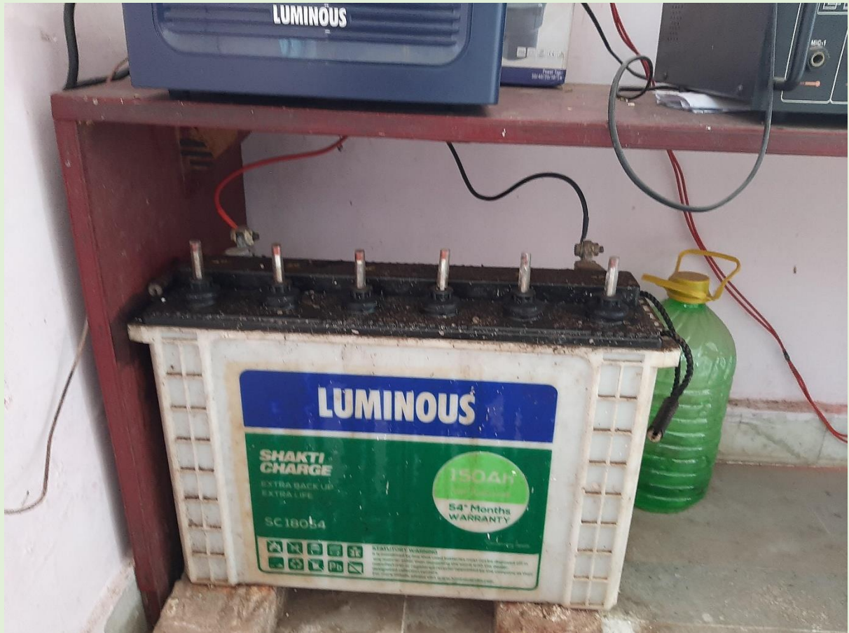
Fig9: Inverter Battery System
