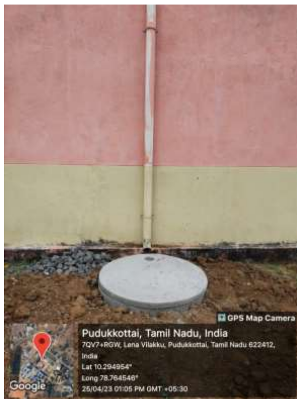
Completely constructed rain water harvesting system at house 1 in Pilivalam
