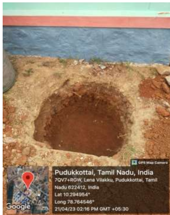
Hole for placing circular rings for the construction of rain water harvesting system
