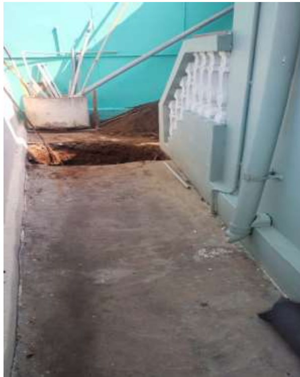
Rain water harvesting system at a house in Melur.
