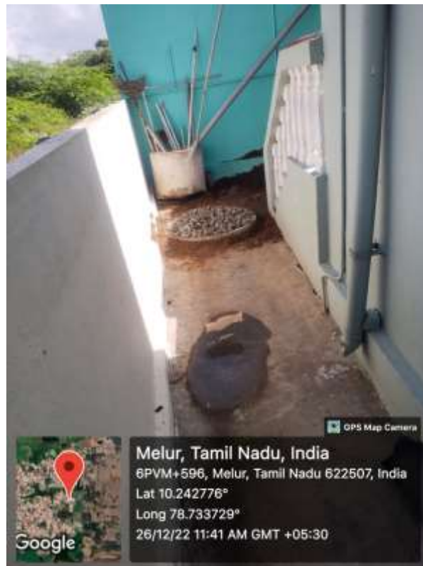
Rain water harvesting system filled with fine aggregate and coarse aggregate
