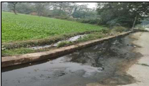
Drainage problem in the village locality
